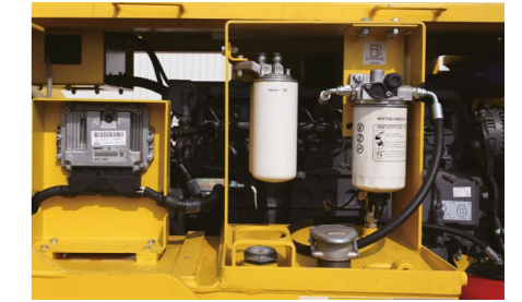
Tier III engine reduces the emissions further. Reduced emission means cleaner air and better working environment in the mine.
